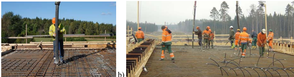
Figure 10: a) Casting SCC on the Nynäsvägen project. b) Casting of normal vibrated concrete.
