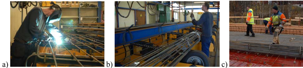
Figure 4: a and b) Manufacturing of carpet reinforcement in a controlled factory environment. c) Placing of carpet reinforcement on the superstructure.
