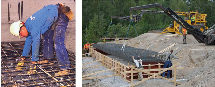
a) b) Figure 11: a) Normal working position for traditional placing of reinforcement. b) Cages of reinforcement placed directly in the form at the Kalix project.
