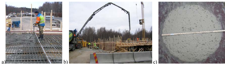
Figure 4: a) Worker using a vibrator for compacting normal concrete. b) SCC being pumped into formwork. c) Slumpflow test on SCC measuring approximately 740mm.
