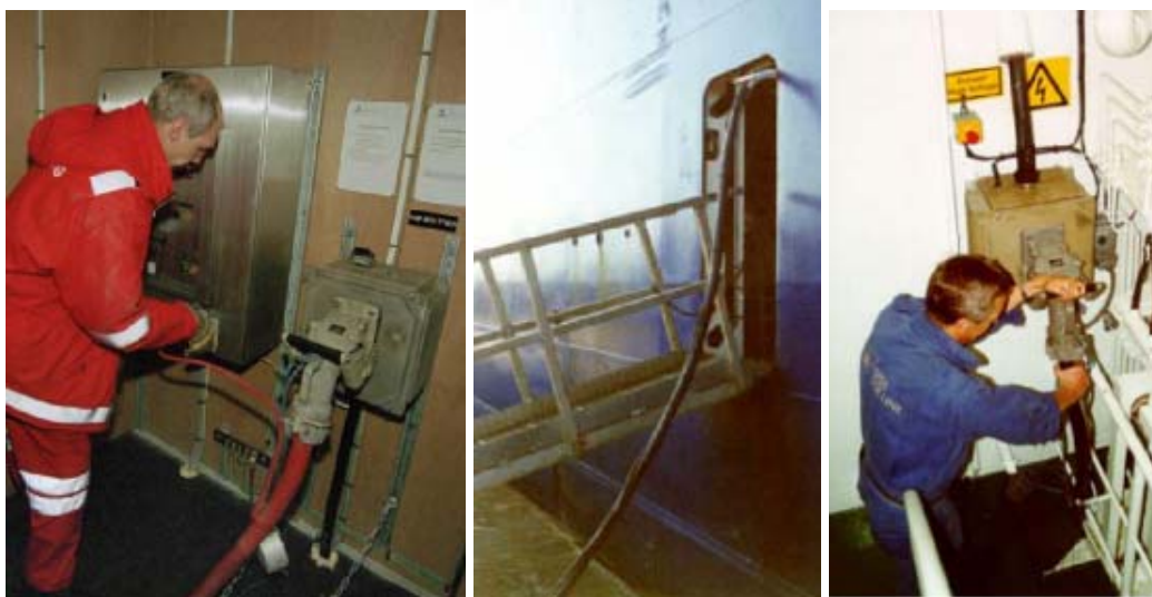
Figure 4 Connection practicalities (Photos: Port of Gothenburg)
